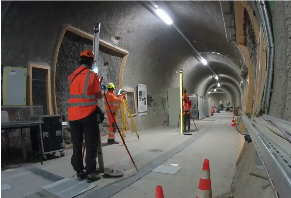
Figure 1: MH: Levelling over the Main Fault in Ga08 (Photo: S. Condamin, swisstopo).
