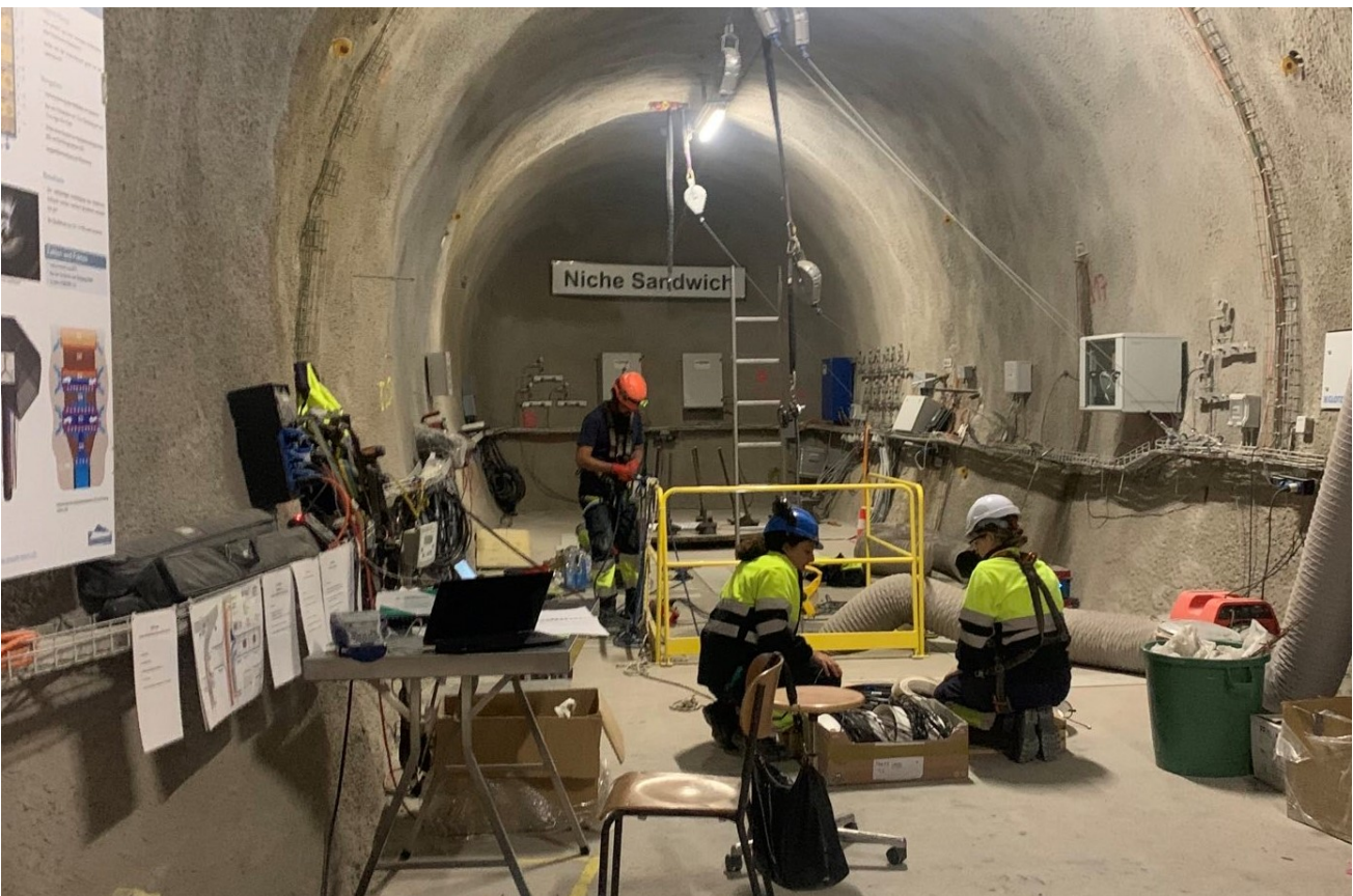
Figure 3: SW-A: The team of AMBERG during the first task of SW-A2 shaft installation and backfilling (Photo: M. Ziegler, swisstopo).
