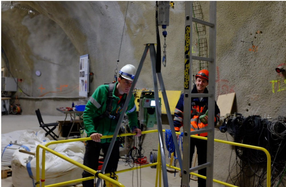
Figure 1: SW-A: G. Graf and P. Maeder preparing for the geodetic measurements inside shaft 1 (Photo: S. Schefer, swisstopo).
