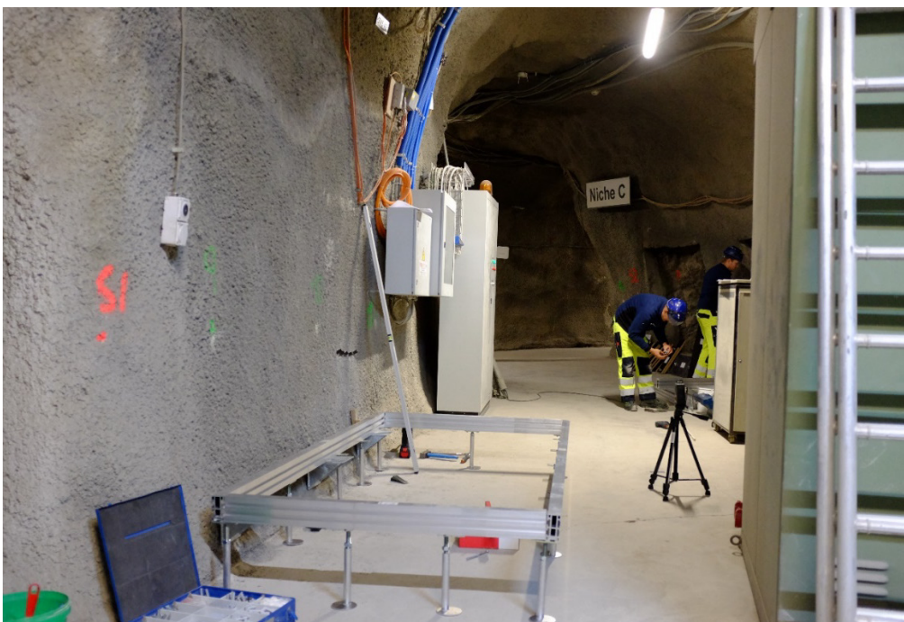
Figure 2: Varia: The frame for the insulating floor is in place. Next week, the new transformer will arrive in Niche C (Photo: S. Schefer, swisstopo).
