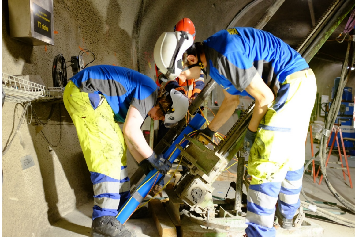
Figure 1: FS-B: Installation of the fibre behind casing inside BFS-B11 (Photo: S. Schefer, swisstopo).
