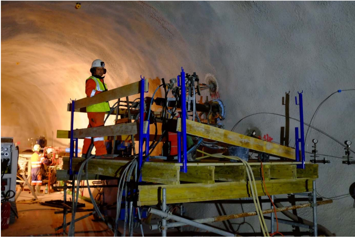
Figure 3: MB-A experiment: S. Sanchez (BGR) on the drilling platform built by the contractor company Zuber (Photo: R. Raselli, swisstopo).
