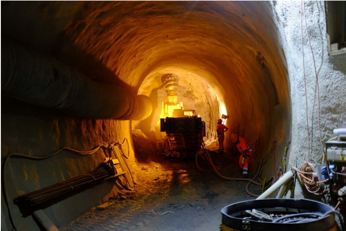
Figure 1: Construction of Gallery 2018: Gallery meter 33 was reached on Friday, August 17 th (Photo: R. Raselli, swisstopo).
