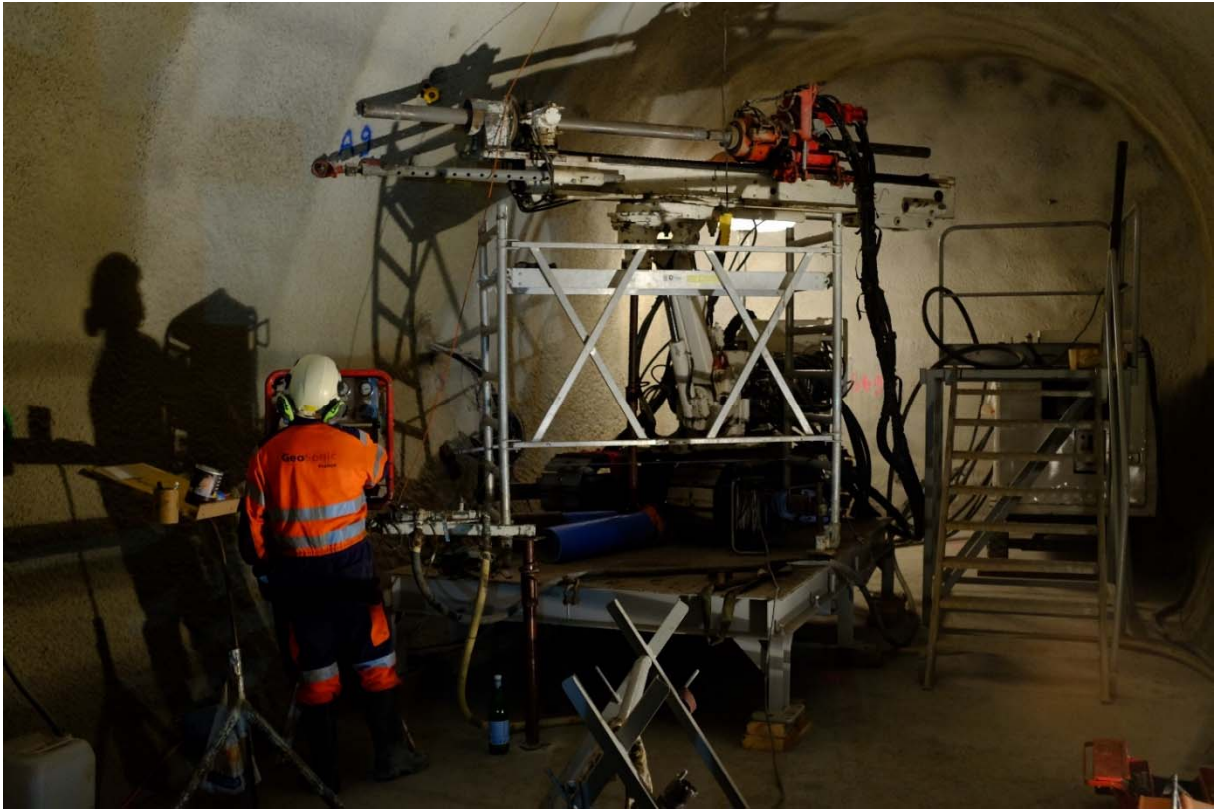
Figure 3: MB-A experiment: Geosonic drilling BMB-A9 with the help of a podium (Photo: R. Raselli, swisstopo).
