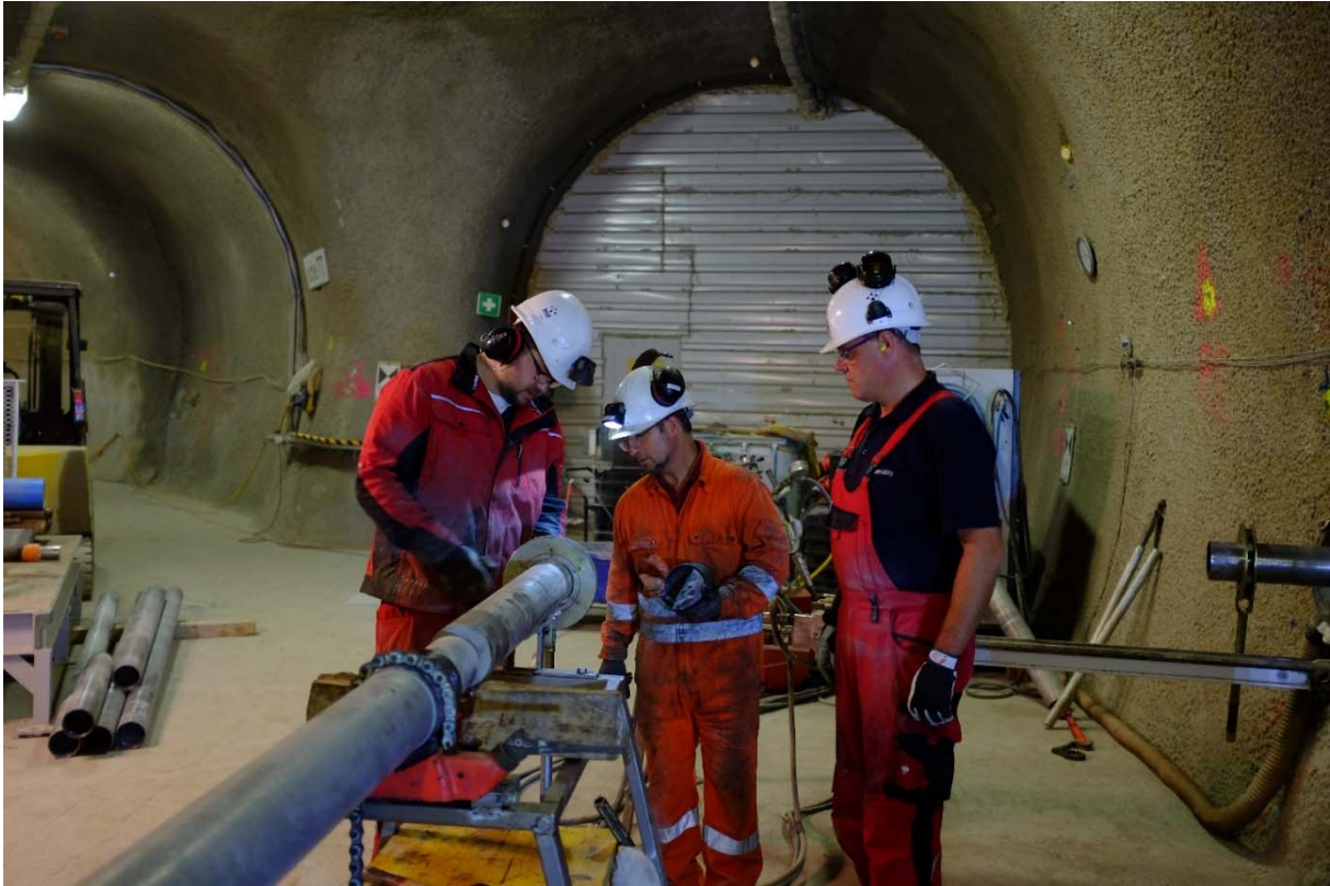
Figure 2: AD experiment: The BGR drilling team drilling borehole BAD-1 (Photo: S. Schefer, swisstopo).
