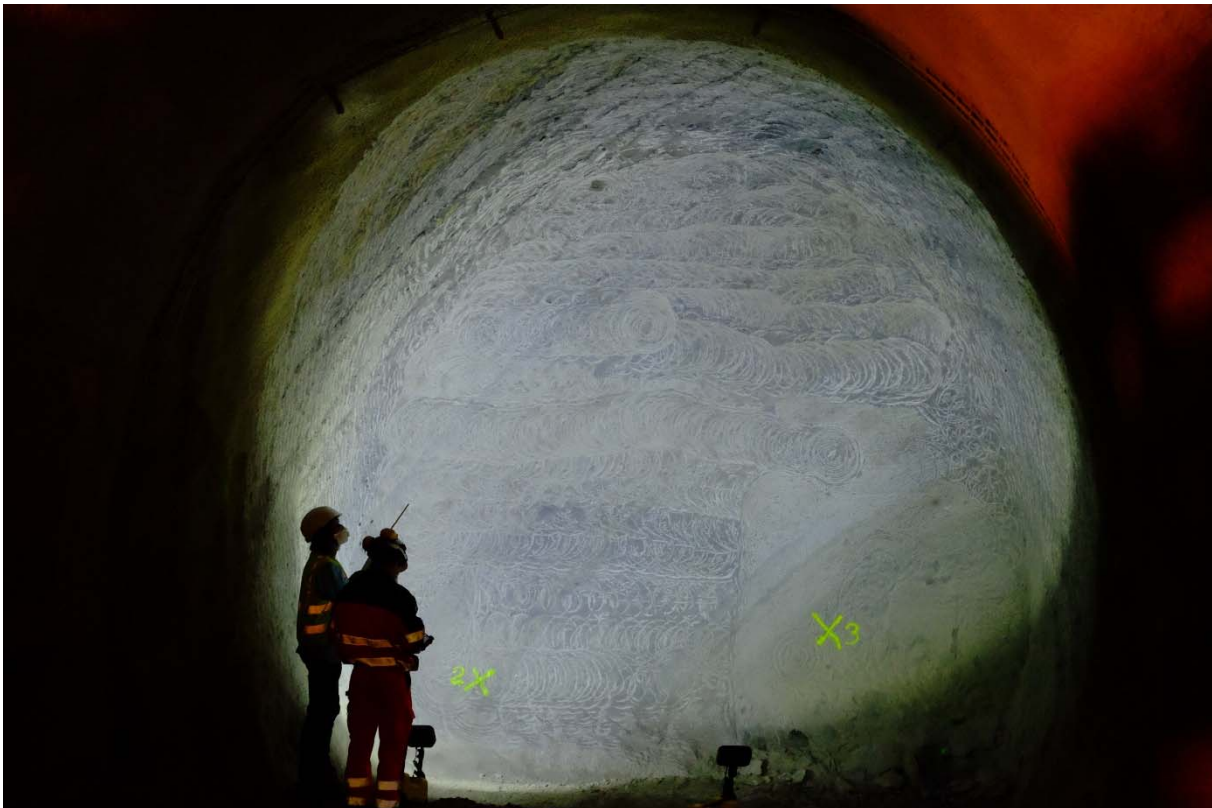
Figure 1: Construction of Gallery 18: The construction of Ga18 continued. Ga18 reached GM 18.0 on Thursday, July 12 th (Photo: S. Schefer, swisstopo). All construction work is stopped during the summer break.
