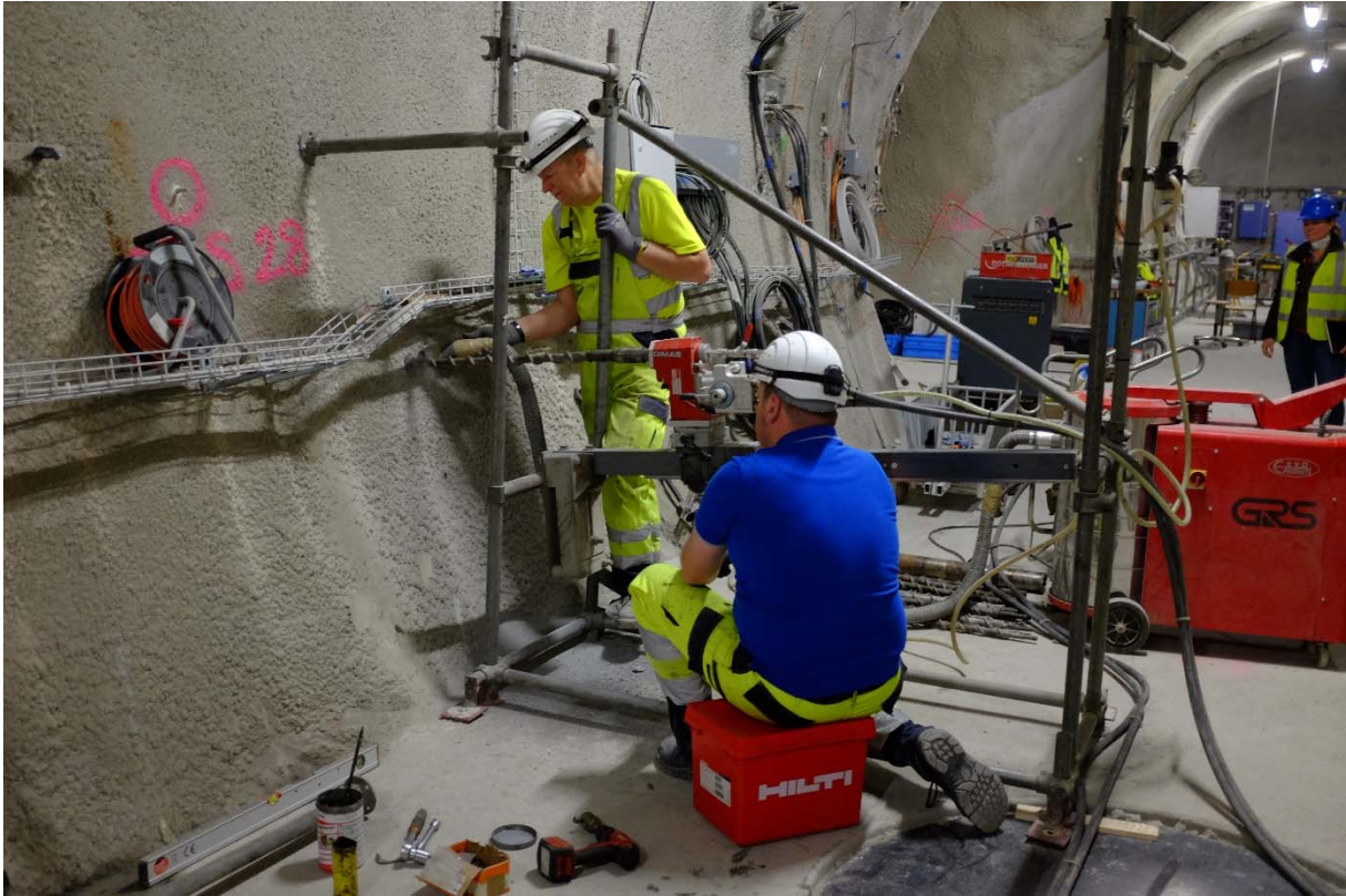
Figure 2: MB-A experiment: M. Komischke and B. Zehle (GRS) installing the drill rig at borehole BMB-A25 (Photo: R. Raselli, swisstopo).
