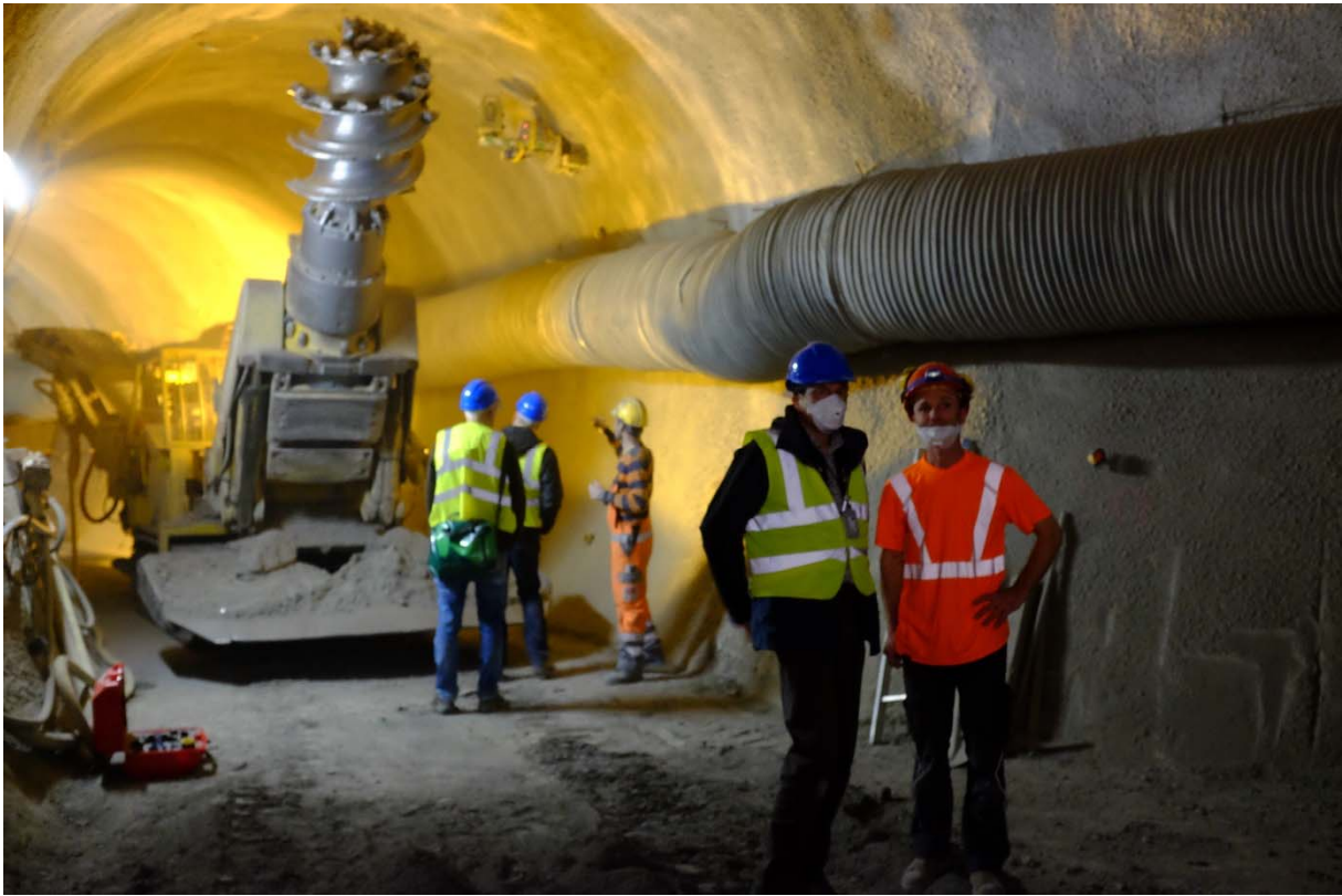
Figure 4: Visits: The company Norbert SA, Géologues-conseils visited the Ga18 construction site together with their guide S. Schefer (swisstopo) to learn about ShapeMetrix and the processing of 3D models (Photo: R. Raselli, swisstopo).
