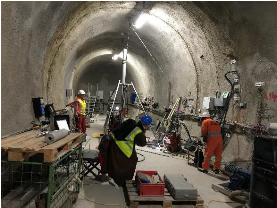
Figure 2: SW-A: D. Novotny and S .Sanchez (BGR) drilling BSW-B26 and photographed by a German journalist (Photo: D. Jaeggi, swisstopo)
