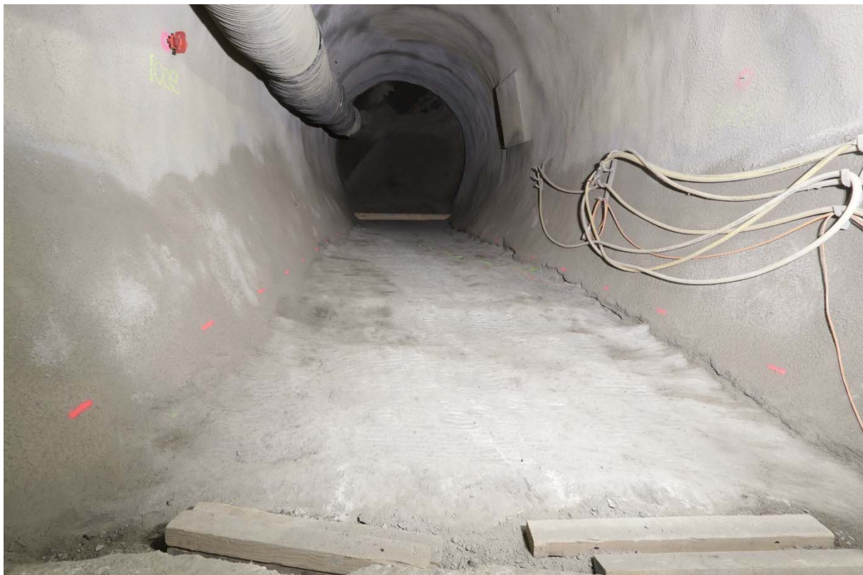
Figure 1: GA18: Gallery 18 is ready for the concrete floor until GM 33.6 (Photo: S. Schefer, swisstopo)
