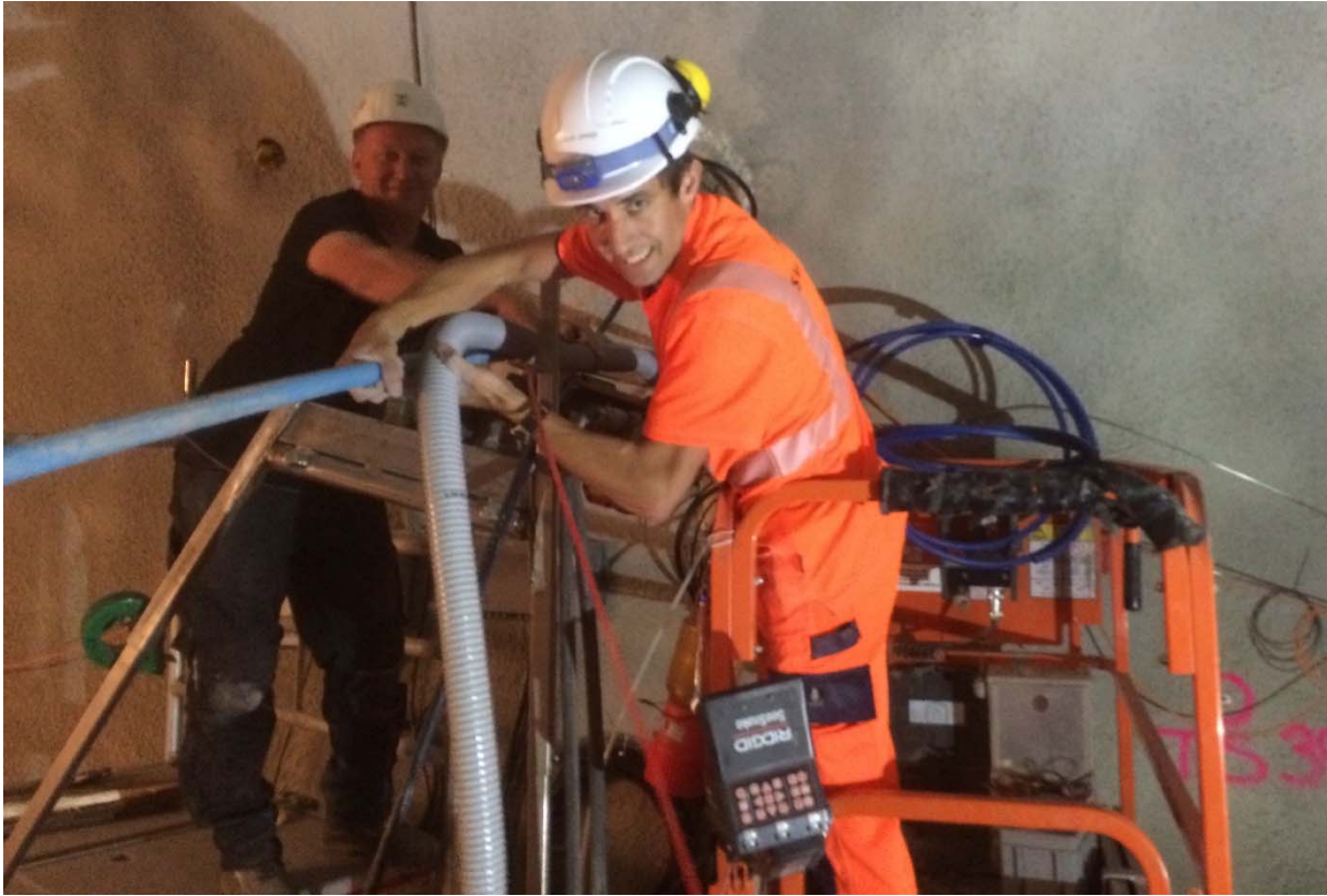
Figure 4: MB-A experiment: D. Jaeggi (swisstopo) and xx (Gloetzi) vacuum-cleaning borehole BMB-A18 before installing the probe (Photo: S. Schefer, swisstopo).
