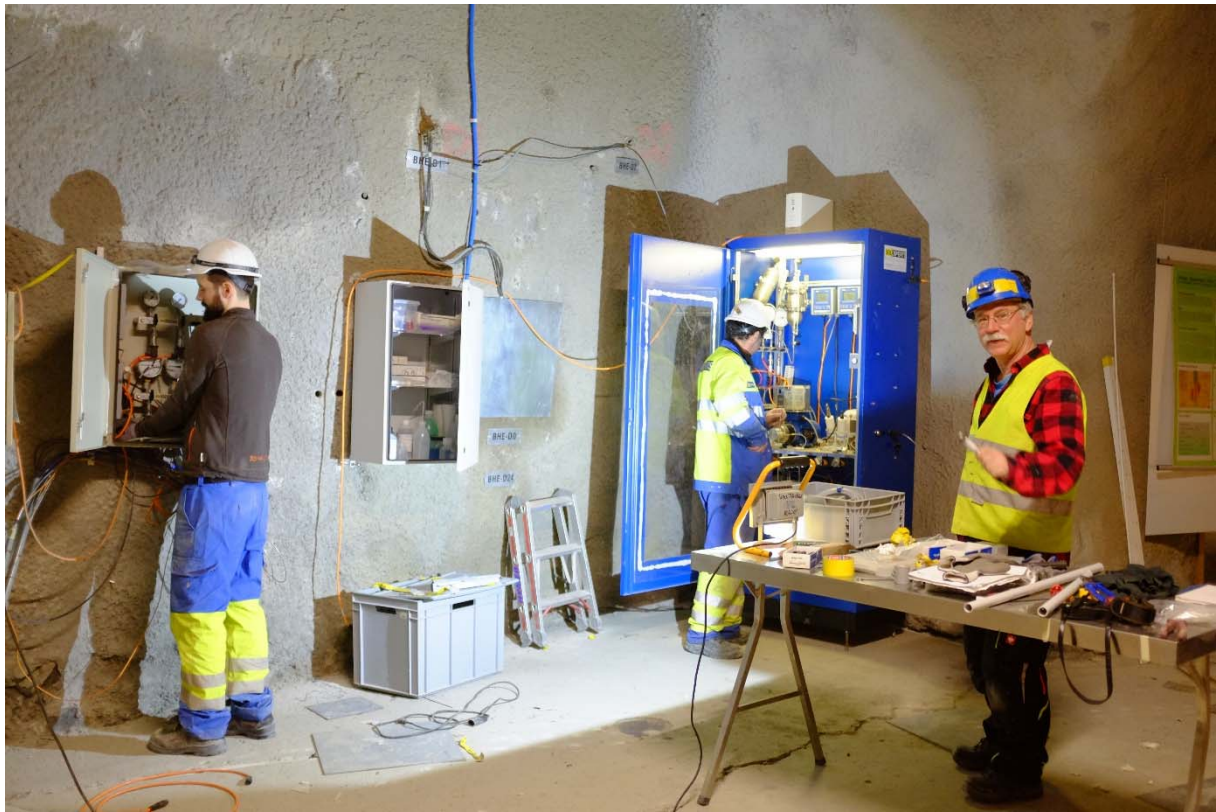
Figure 2: CI-D: U. Mäder (University of Bern) and the team from Solexperts relocating the CI-D cabinet to its original location in niche HE-D (Photo: R. Raselli, swisstopo).
