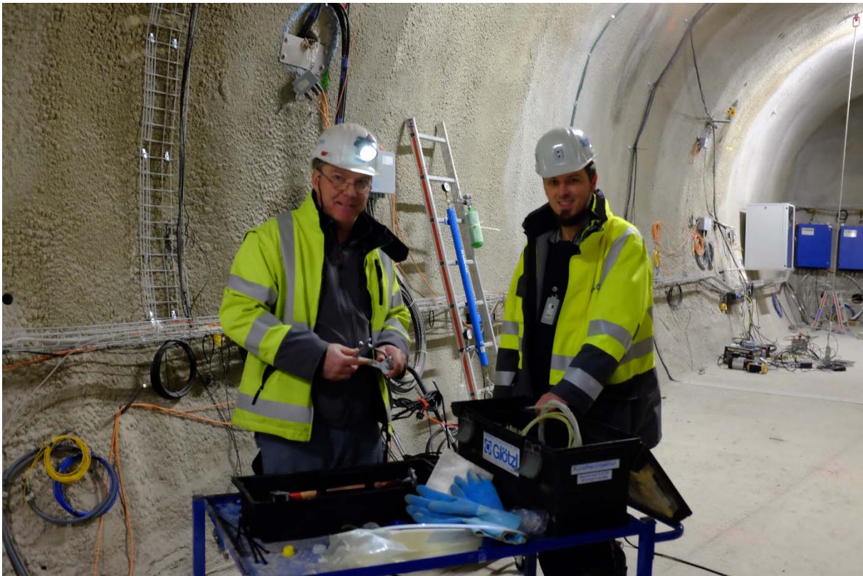
Figure 1: MB-A: T. Kostreva and F. Herfurth (Glötzi) during the installation for the resin injection (Photo: R. Raselli, swisstopo).
