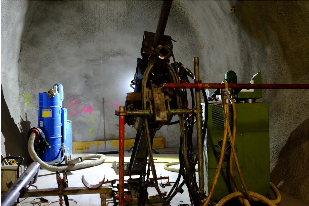
Figure 2: GC-A experiment: H. Gutgesell (behind the green control panel) drilling borehole BGC-A1 in the pre-Niche North of Niche 2 (southeastern prolongation of the DR niche) (Photo: R. Raselli, swisstopo).
