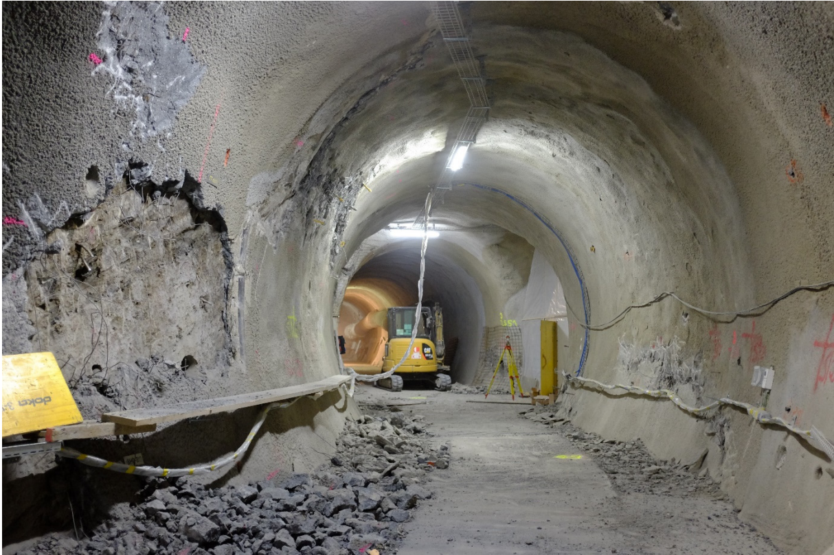
Figure 1: Ga18: Repairing of the shotcrete in Niche TT and Ga 18 (Photo: S. Schefer, swisstopo).
