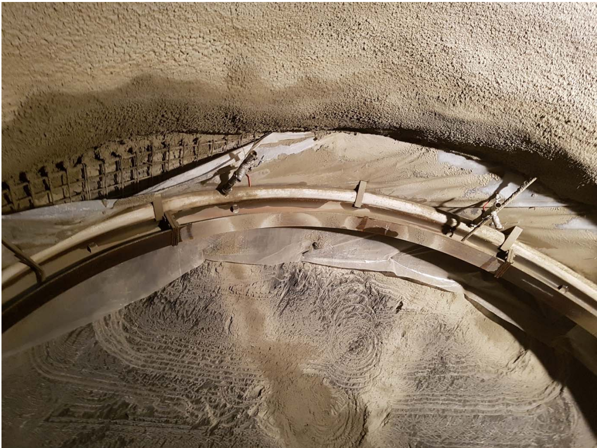
Figure 3: TS experiment: First bullflex installed in section TS-2 (Photo: F. Burrus, GGT).
