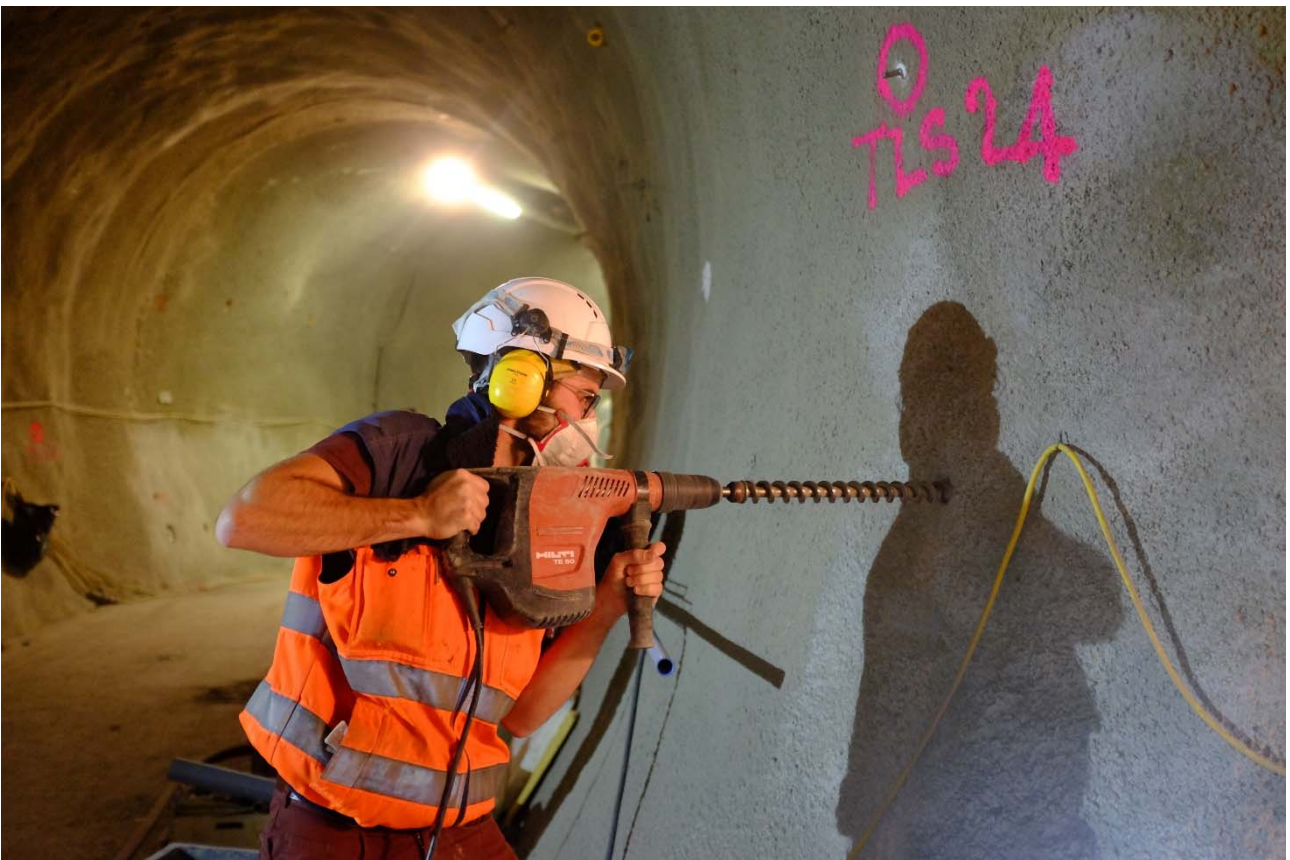
Figure 4: Safety: M. Ringeisen (swisstopo) drilling holes in shotcrete in the niches 7 & 8 to check and verify the thickness of the shotcrete (Photo: S. Schefer, swisstopo).
