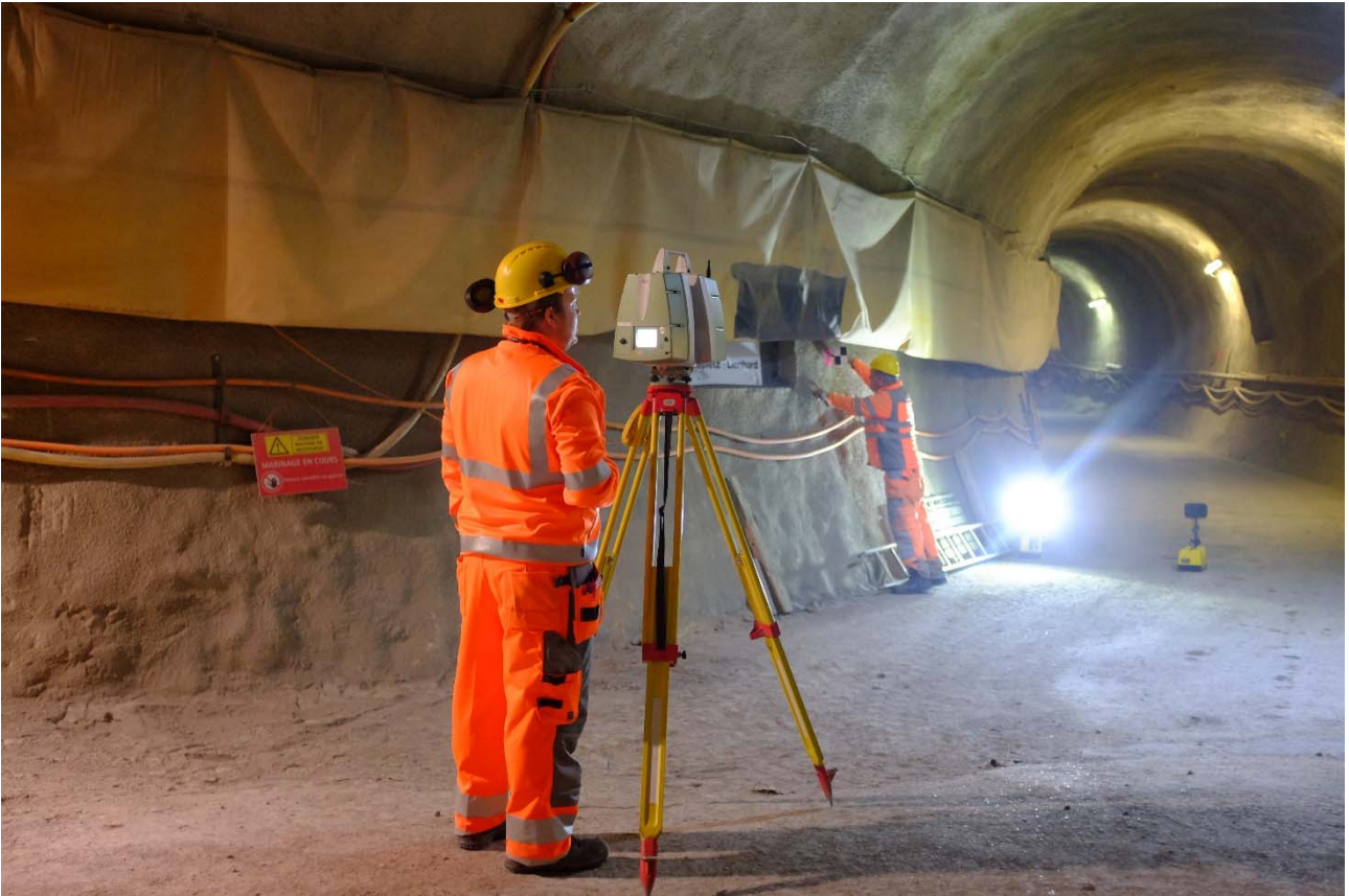
Figure 1: Gallery 18: N. Philipposien and Q. Bobillier (Sigeom SA) preparing the next laser scan (Photo: S. Schefer, swisstopo)
