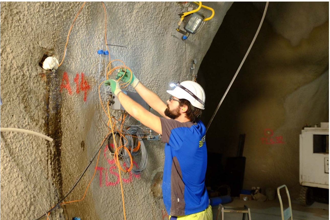
Figure 2: MB-A: L. Schwab (Solexperts) connecting pressure transducers to the Geomonitor system (Photo: S. Schefer, swisstopo).
