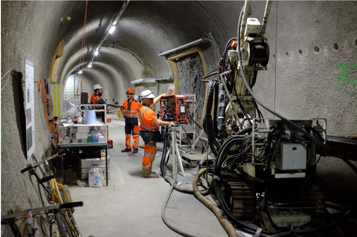
Figure 1: CS-D: The drilling company GeoSonic drilling borehole BFS-B4 (Photo: R. Raselli, swisstopo).
