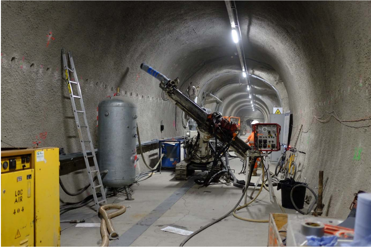
Figure 3: SI-A: GeoSonic drilling boreholes BSI-A17 to BSI-A32 in Gallery 08 (Photo: R. Raselli, swisstopo).
