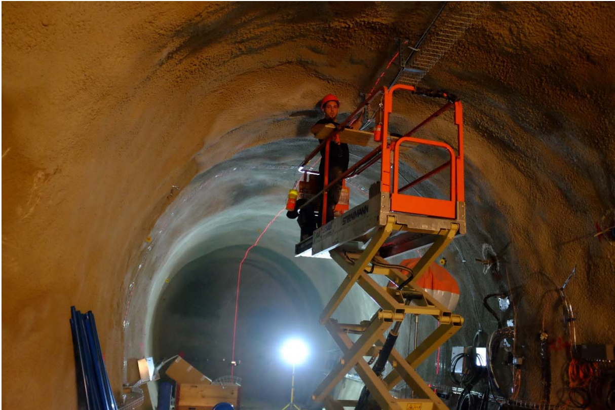
Figure 2: CS-D: A. Rinaldi (ETHZ) marking the spots where geophones will be installed. (Photo: R. Raselli, swisstopo).
