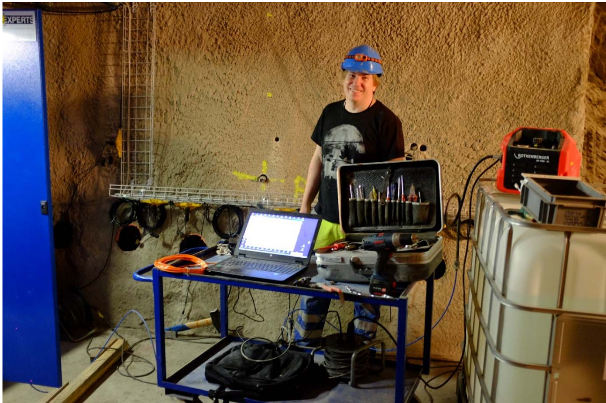
Figure 3: CS-D: J. Gisiger (Solexperts) performing the saturation of boreholes BCS-D1 and BCS-D2 (Photo: R. Raselli, swisstopo).
