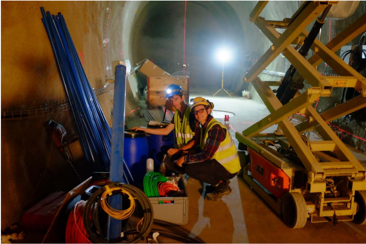
Figure 1: CS-D: Q. Wenning and M. Grab (ETHZ) preparing the installation of several geophones in Niche 8. (Photo: R. Raselli, swisstopo).
