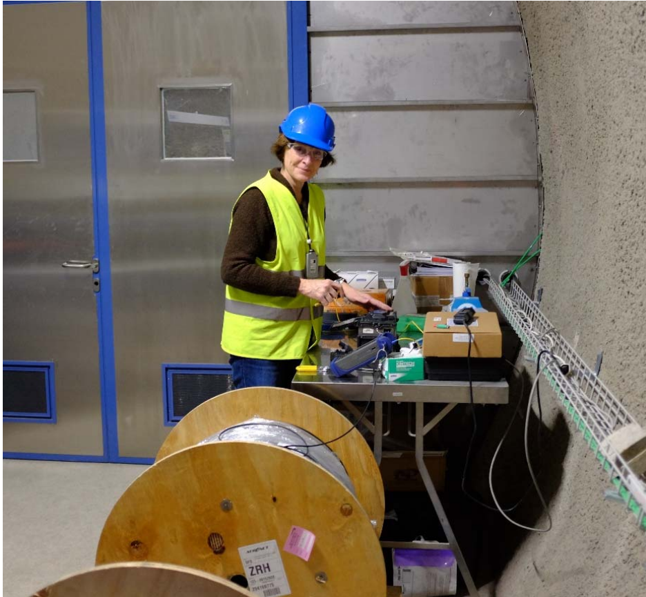
Figure 2: FS-B: M. Robertson (LBNL) was on site, preparing for the fiber optical installations in the borehole BFS-B5. She spliced pigtails onto both ends of the cables in preparation for downhole installation (Photo: R. Raselli, swisstopo).
