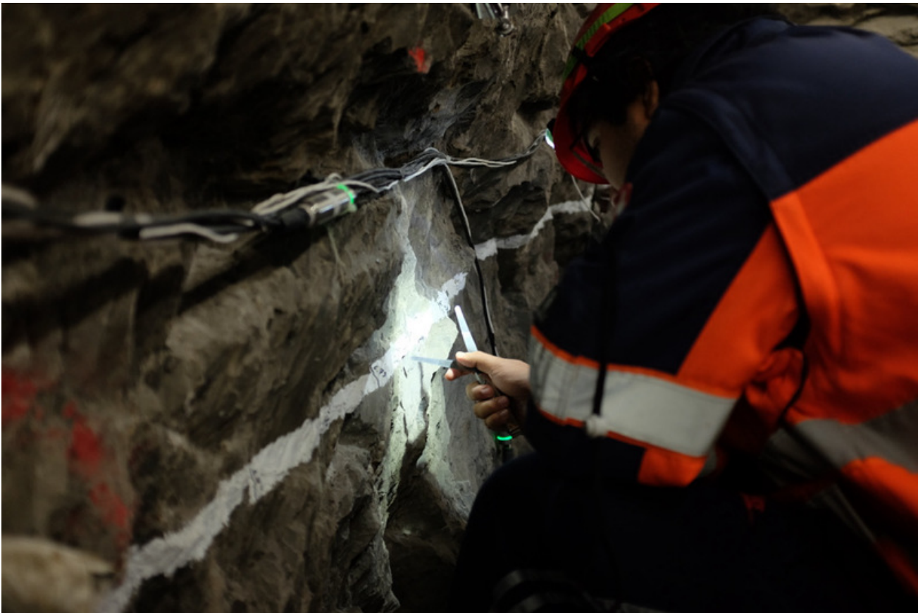
Figure 1: CD-A: L. Borgeaud (swisstopo) measuring the crack apertures along the open niche (S. Schefer, swisstopo).
