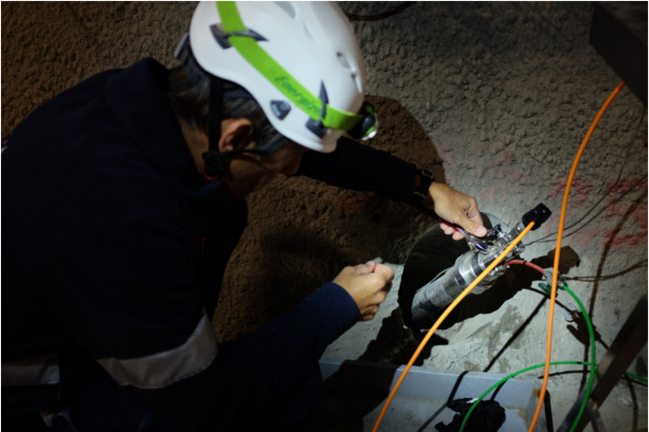
Figure 3: SW-A: D. Jaeggi (swisstopo) installing the pressure transducer (A. Grignaschi, swisstopo).
