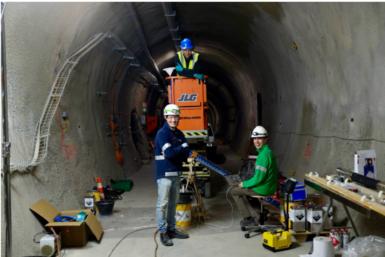
Figure 1: CL: M. Ziegler, A. Grignaschi, J. Windisch (swisstopo) with S. Czerner and T. Fritsche (ZHAW) prepare the setup for the resin injection (A. Grignaschi, swisstopo).
