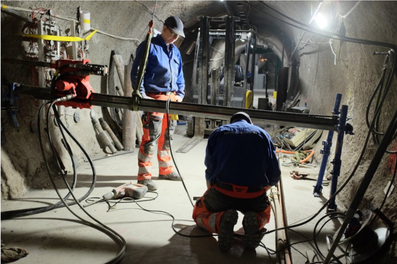
Figure 1: HE-E: Installation of the drill rig for HE-E4 inside Ga98 (J. Windisch, swisstopo).
