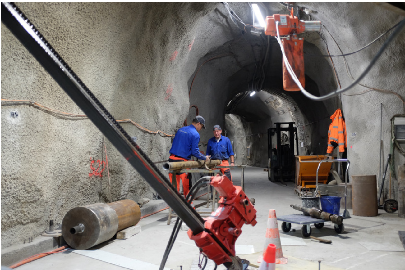
Figure 2: CI-D: Preparation of the core barrel for the overcoring (S. Schefer, swisstopo).
