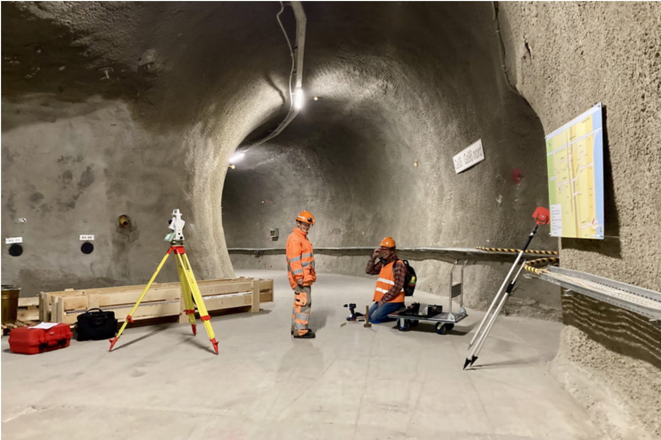
Figure 1: BIM: Implanting one of the many fixpoints along the tunnel axes (S. Schefer, swisstopo).
