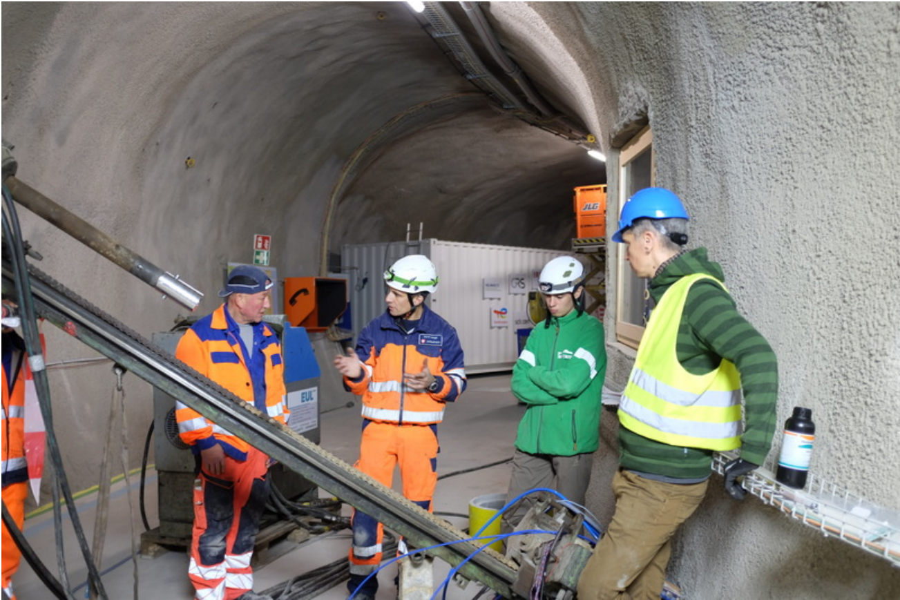
Figure 4: CL: Many sensor cables and tubes had to be neatly placed for the installation (S. Schefer, swisstopo).
