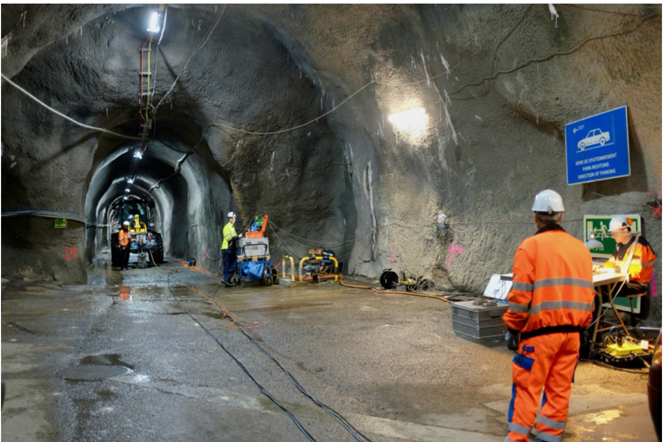
Figure 4: SI-B: The team from GFZ acquiring seismic data in the Safety Gallery (A. Grignaschi, swisstopo).
