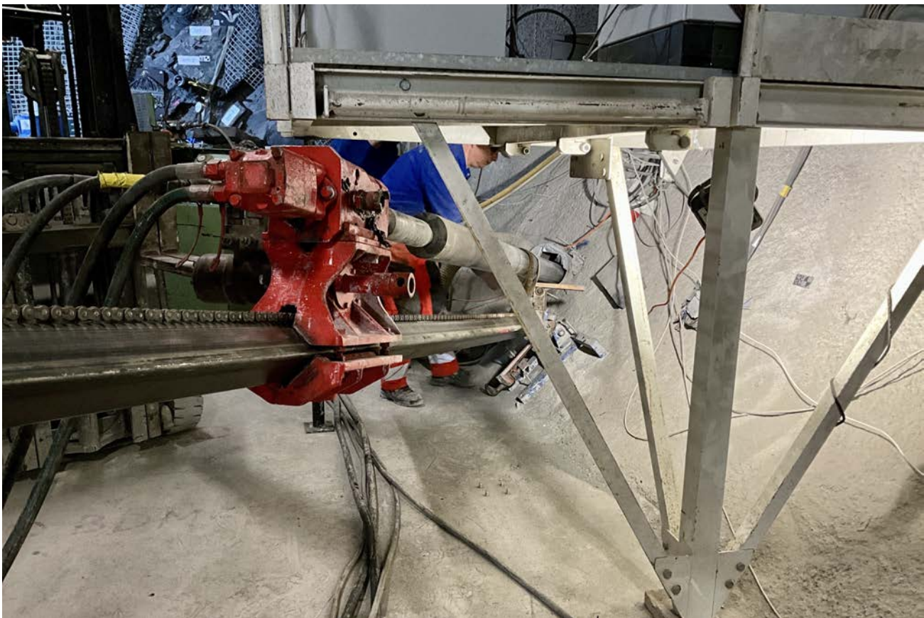
Figure 2: PF-A: Installed rig on BPF-A1 and drilling in tight space underneath the heater controllers of HE-E (J. Windisch, swisstopo).
