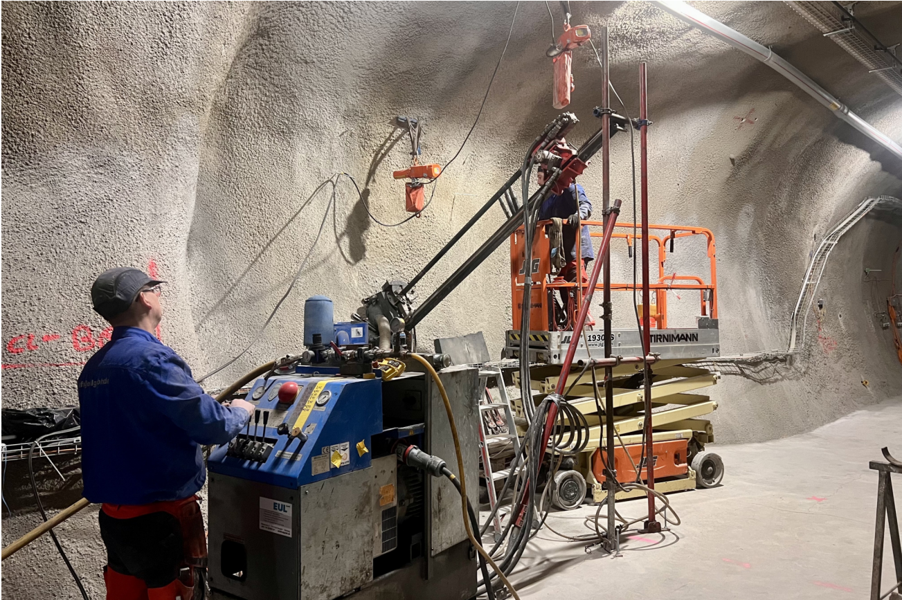
Figure 1: CL: Drilling of BCL-5 in Niche CL. This is the first of four monitoring boreholes (J. Windisch, swisstopo).
