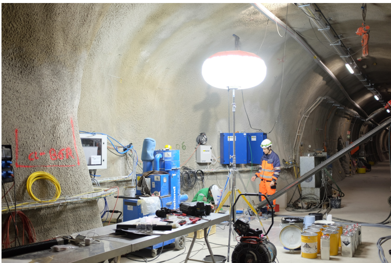
Figure 4: CL: The resin is injected with a pump. A lot of cleaning is involved... (S. Schefer, swisstopo).
