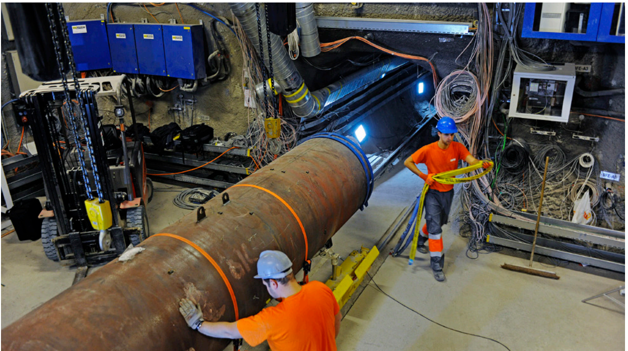
Figure 5: Installation of a canister in the “Full-Scale Emplacement Experiment” on a scale of 1:1, under the lead of NAGRA. Instead of radioactive waste, the canister contains a heating element to simulate waste heat.
