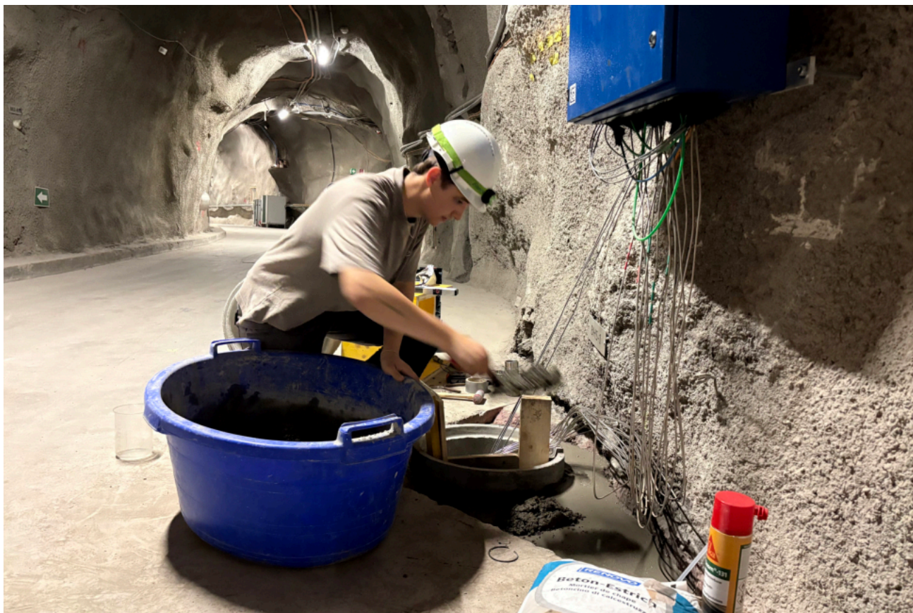
Figure 1: HS: N. Rentsch pouring the last layer of concrete around BHS-1 (S. Schefer, swisstopo)
