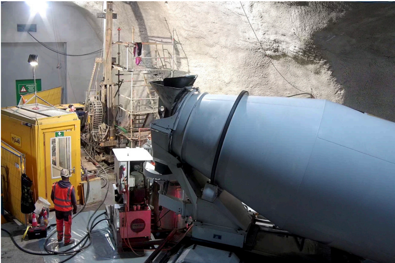
Figure 1: DB-B: A new powerful pump to accomplish the challenging cement job (S. Schefer, swisstopo)
