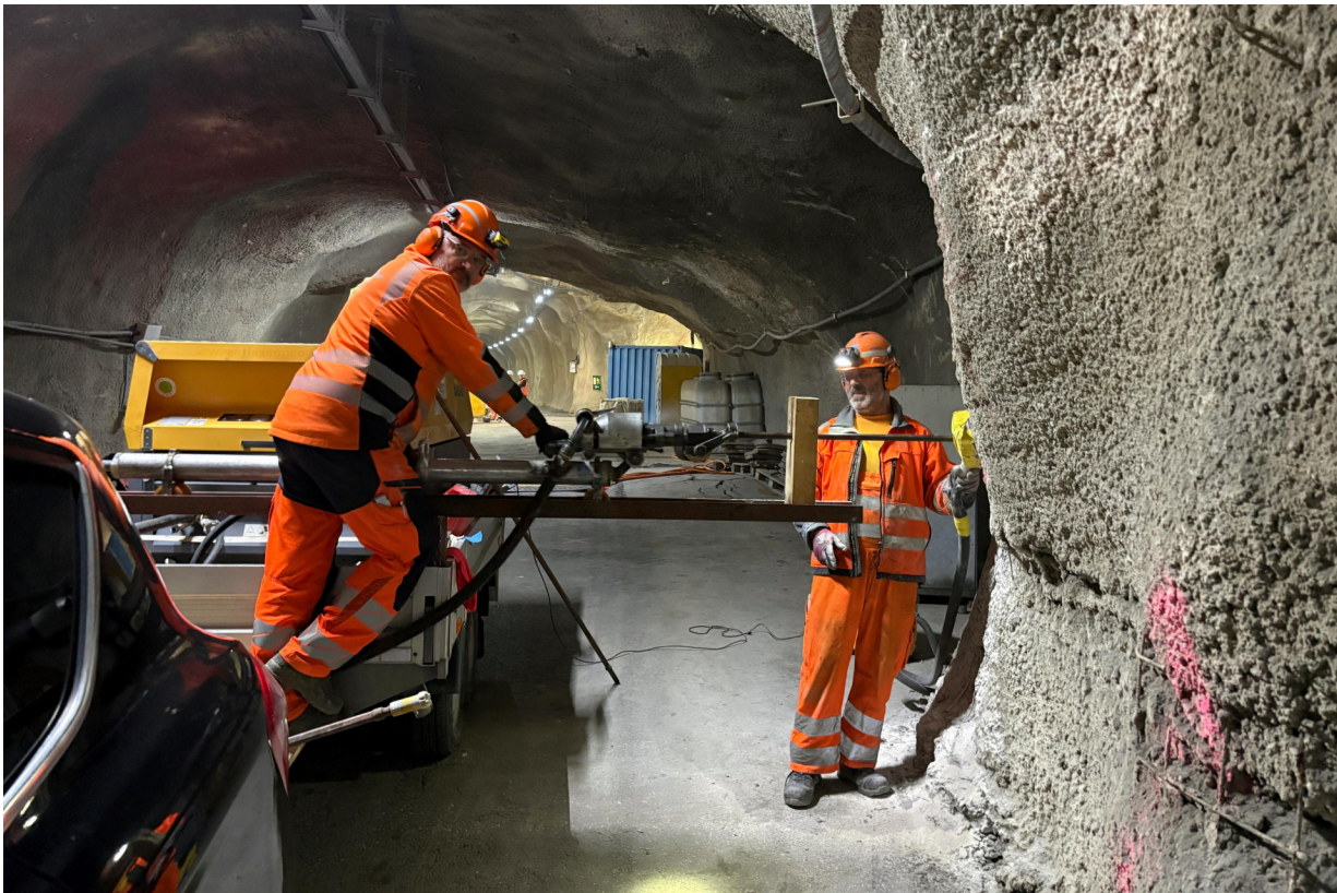
Figure 2: SI-C: Drilling for the seismic campaign started next to Deborah (S. Schefer, swisstopo)
